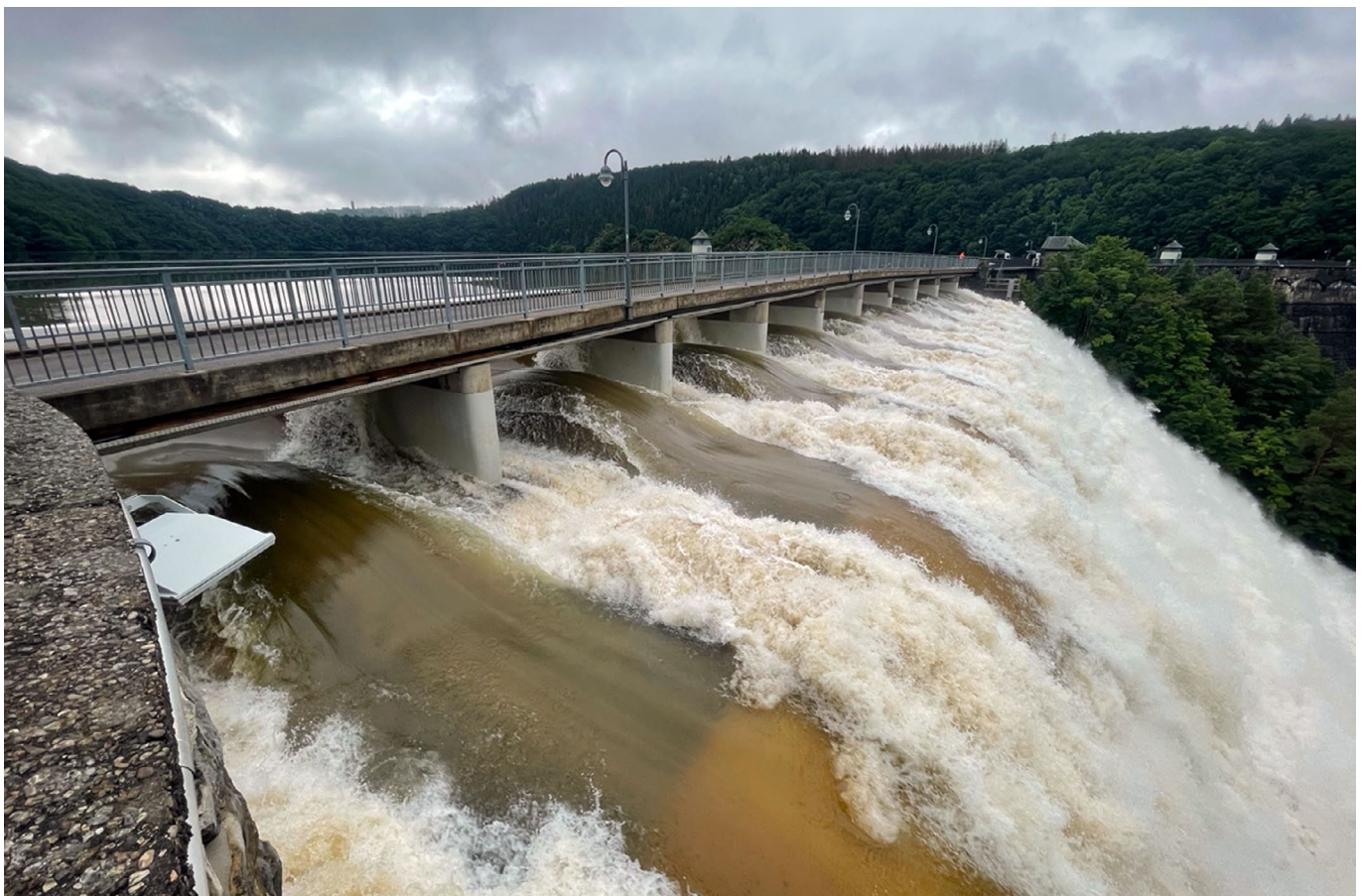
Figure 2 | Flood discharge (specific discharge approximately 3.5 m 3 /s) at Urft dam in the morning of 15 July 2021, the design discharge of 3.17 m 3 /s for a 10,000 year flood was exceeded, leading to significant overtopping of spillway sidewalls.
