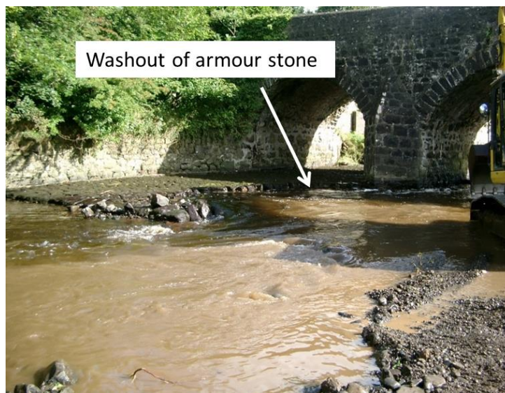
Figure 8. Supercritical flow immediately downstream of this arch bridge washed out armour stone placed there, and then (via a head-cutting mode) eroded the downstream bed; Co. Antrim, Northern Ireland
