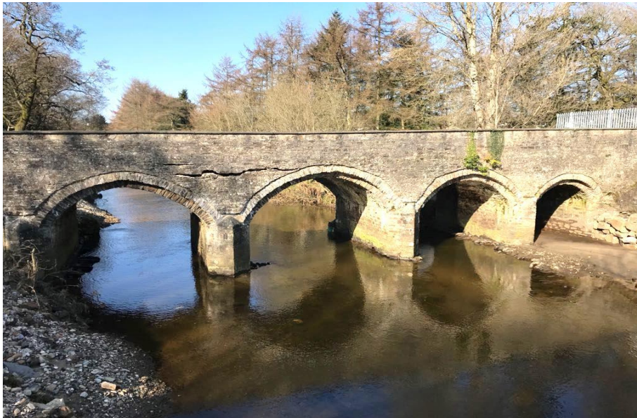
Figure 1. Scour at the front of the central pier led to scour-induced failure of an arch bridge (Ballynameen Bridge) over the River Faughn near Cladys, Northern Ireland. (View looking from upstream of the bridge)
